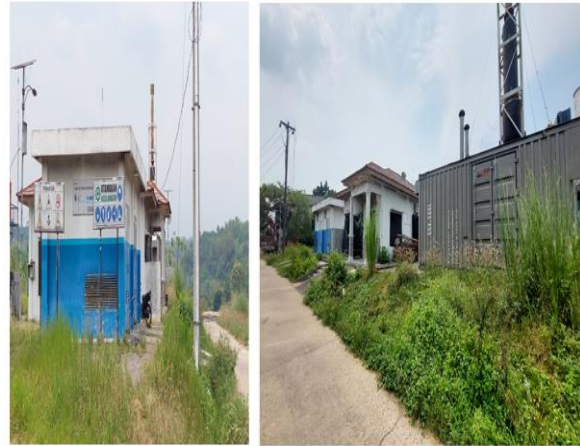
Figure 6. Power Plant Installation with Biogas Technology (Methane Gas)
